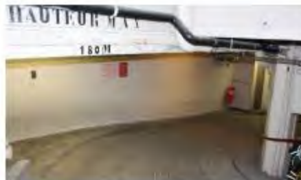
3. Basement car park: height access limited
