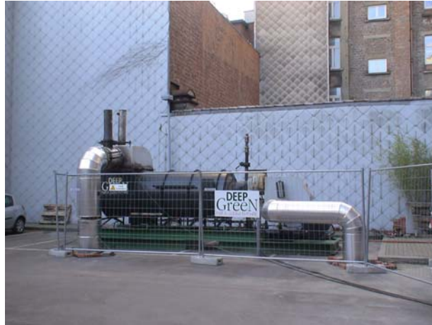
Fig4. Thermal oxidizer installed outside, on the ground floor, just above the polluted area
