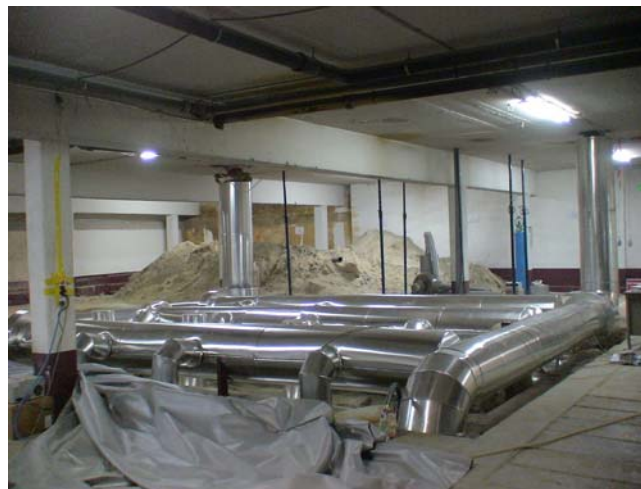
Fig 3bis. Pipe network on the polluted area
