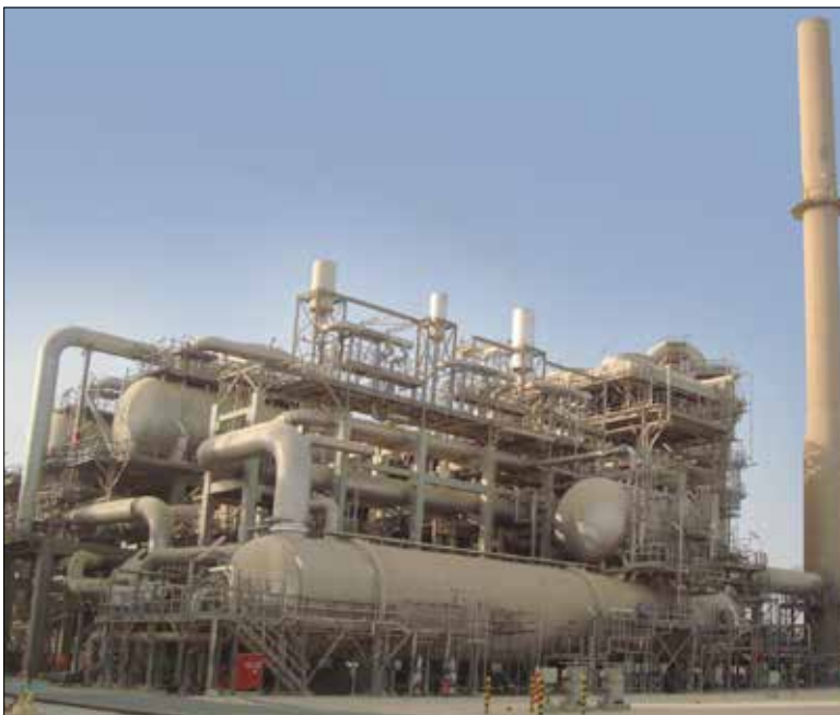
Figure 3 Sulphur recovery unit (SRU) tail gas thermal oxidiser with a fire tube-style waste heat boiler. This unit is designed for a total 75 MW heat release
