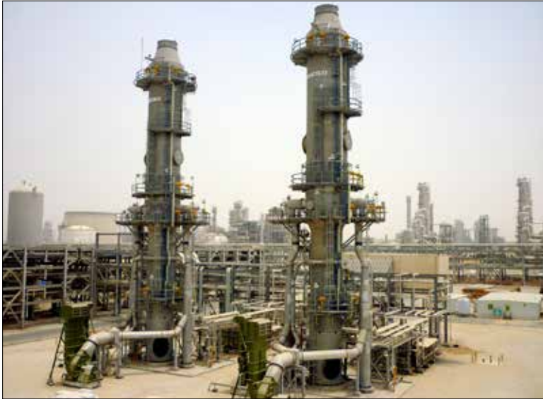
Figure 2 Two vertical low-NOx thermal oxidisers used for NOx reduction
