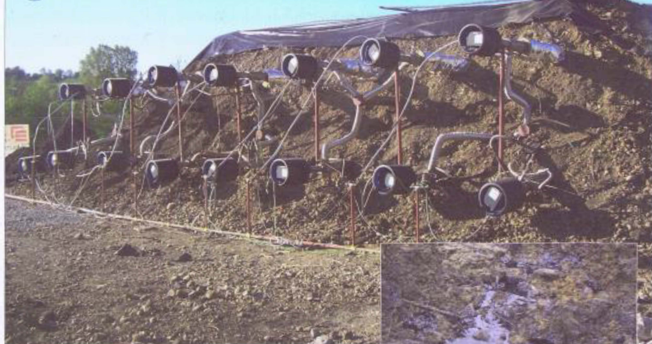
Above: NSR© Industry; Inset: Creosote contaminated soil
